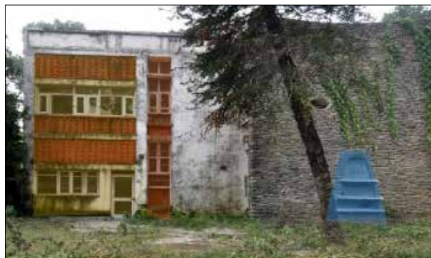
Figure 2.8: The derelict state of the Pierre Jeanneret house front before its restoration; Source: Ar. Deepika Gandhi
