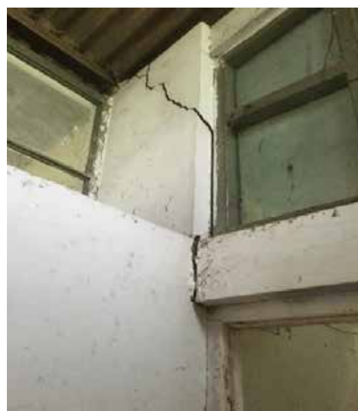
Figure 2.12: Structural cracks at the Le Corbusier Centre; source- Ar. Deepika Gandhi
