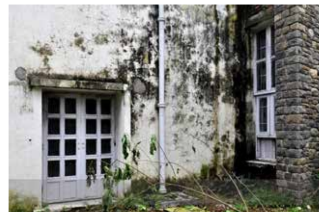
Figure 2.9: The exterior surfaces of the house taken over by algae deposits; Source: Ar. Deepika Gandhi
