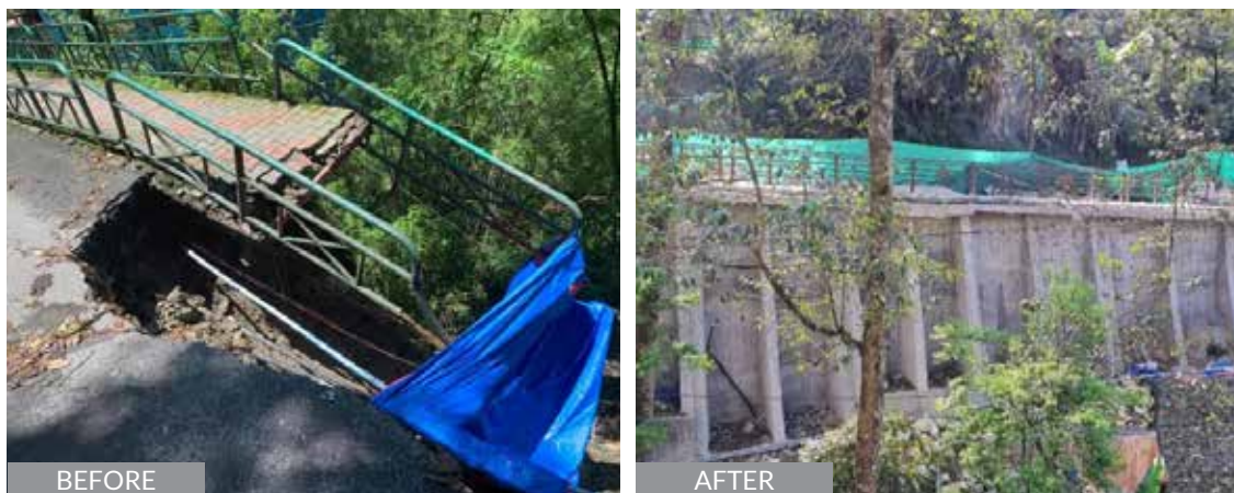
Figure 18: Old overhanging footpath (left) & new overhanging footpath on plumb concrete retaining walls Source: DPR, 2018 (left) & IIT Kharagpur Survey (right)
