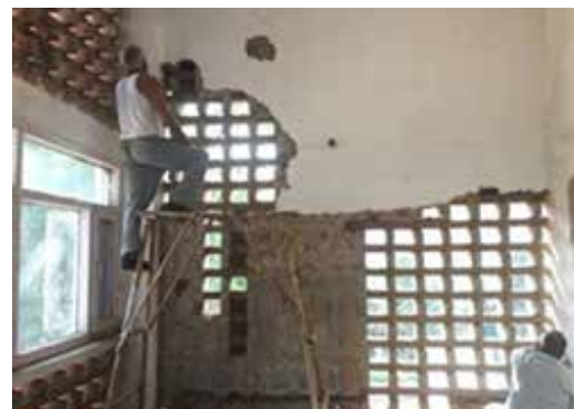
Figure 2.29: Plaster removed to reveal original brick jaali on the encroached veranda on the first-floor level Source: Author
