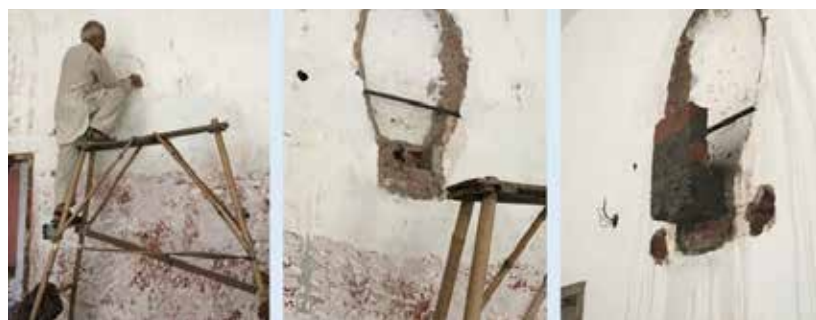
Figure 2.26: The process of restoring the light niche that had been covered up with brickwork and plaster; Source: Ar. Deepika Gandhi
