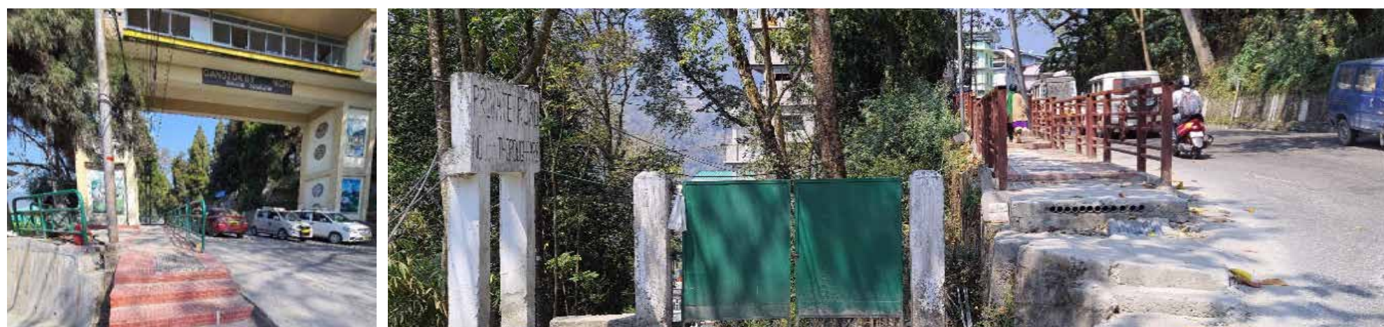
Figure 24: Stairs for accessing the footpath without railings Source: IIT Kharagpur Survey
